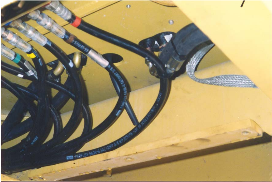
View showing underside of evaporator area with hose assemblies and drain tubes.
